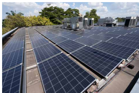
Installation of a 671 m 2 solar array on the rooftop of the Petit-Pont commercial building (business district), with an average output of approximately 380 kWh/day
